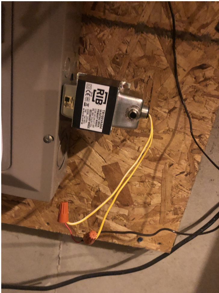
120VAC to 24VAC transformer, 96VA
