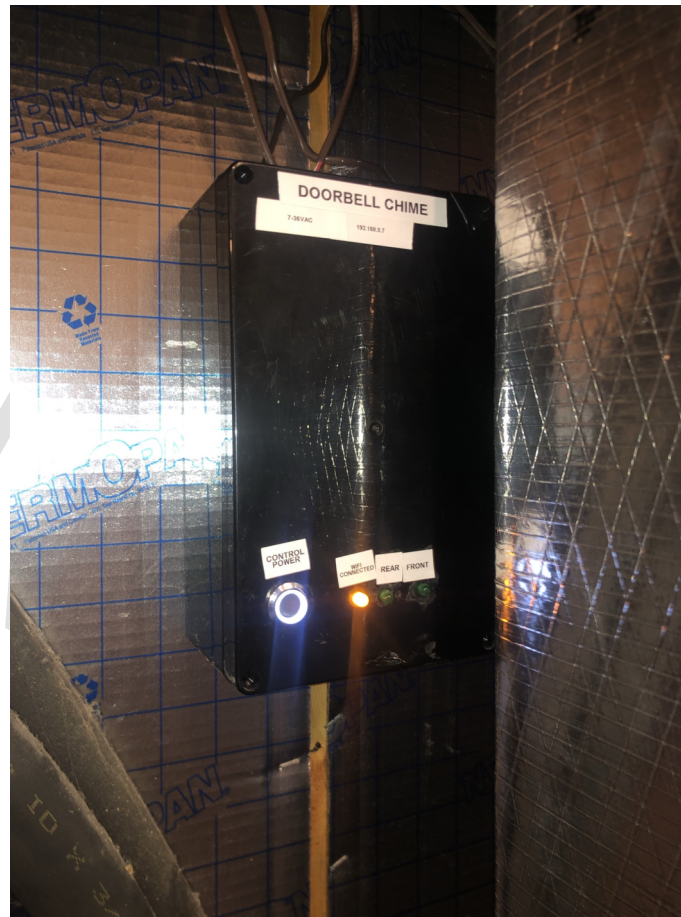
Completed Device mounted in final location Closed Cover shows control power switch (ring lit while powered on), Wi-fi status light, and the Front and Rear Door Status lights.
